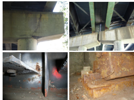
Figure 2. Typical findings at the Wayne Bridge
